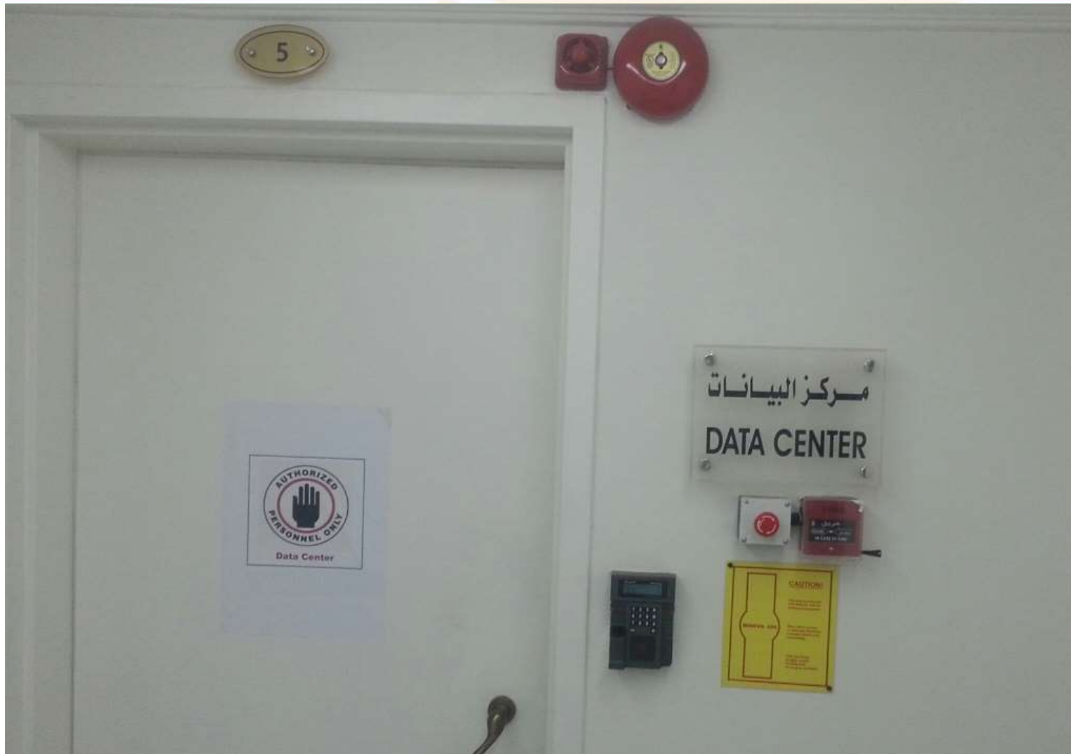
Access Control and Alert Systems for Data Centers
